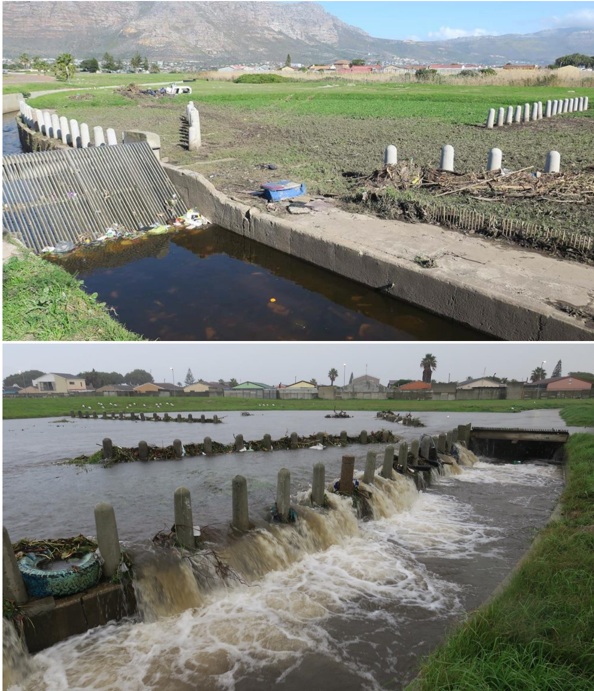
Figure 4. An inclined grid screen installed by the City of Cape Town municipality on a canalised section of river leading into Zandvlei, Cape Town (top). If serviced regularly, this system works fairly well under low to moderate flow conditions, but rapidly becomes blocked during high flow conditions, requiring an overflow basin with bollards to trap larger debris items.
