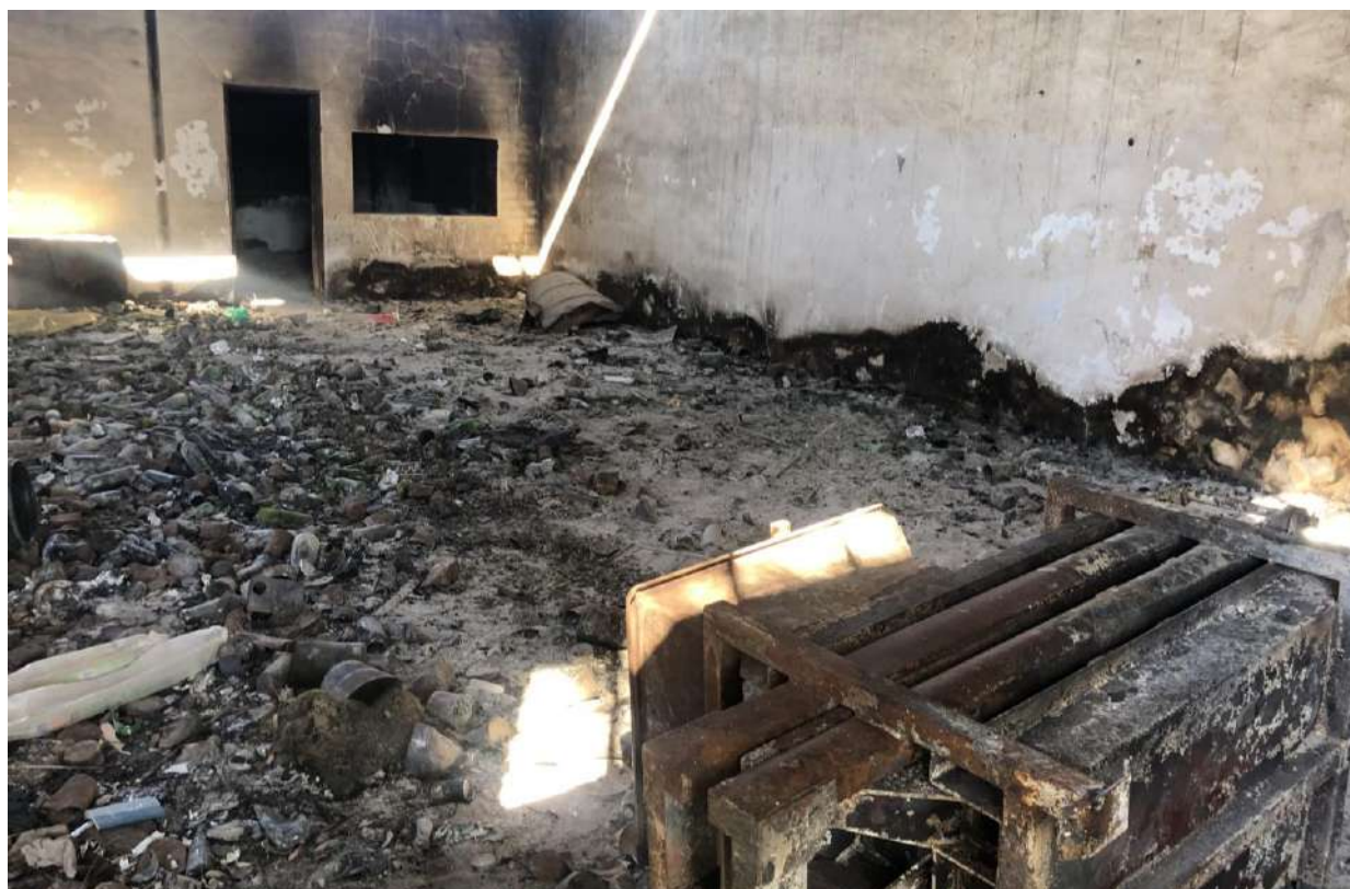
Figure 61: Recyclables, building and sponsored hand baler destroyed in the fire in Philippolis Source: Researchers
